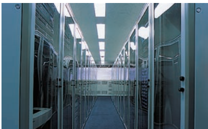
Five data centers located nationwide provide various services
